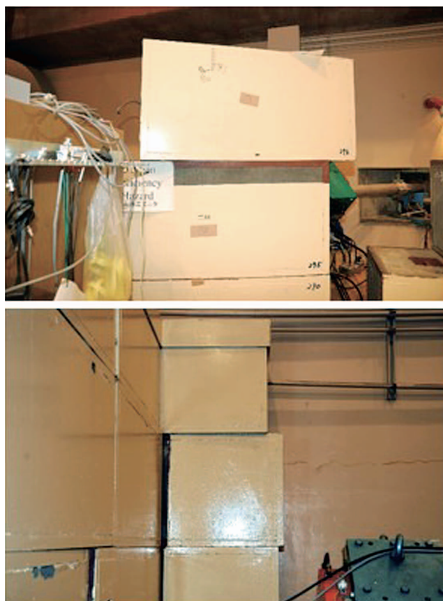
Fig. 8. Mismatch between shielding blocks.
