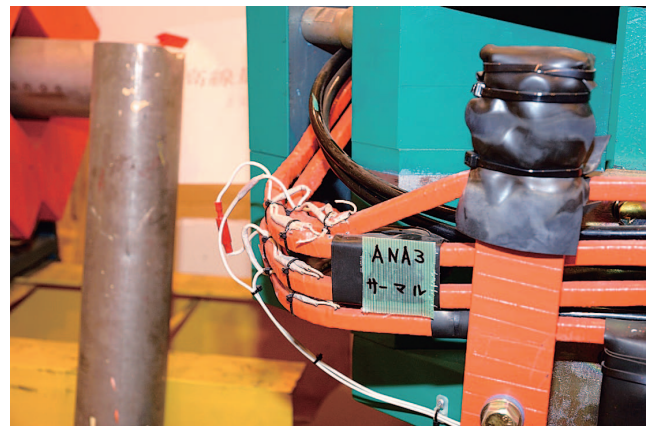
Fig. 5. Electromagnet damaged by falling object.
