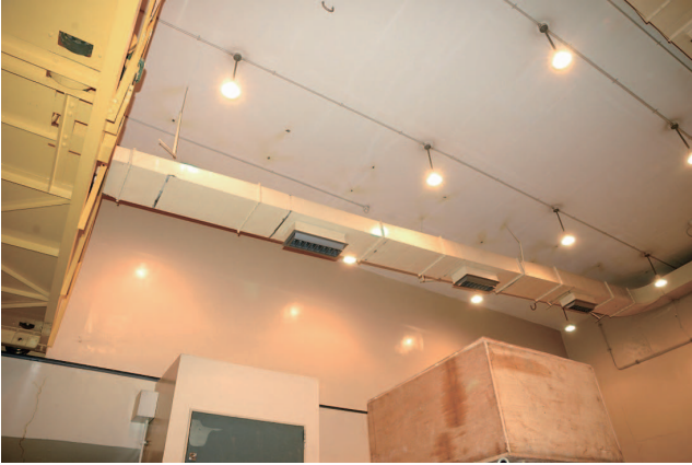
Fig. 6. Ventilation duct that fell onto the ceiling crane. In the electromagnet room, the hanging columns of the ventilation duct fell, and the duct dropped. The duct stopped on the ceiling crane and did not fall onto the beam line. Consequently, further damage of the beam line was prevented.
