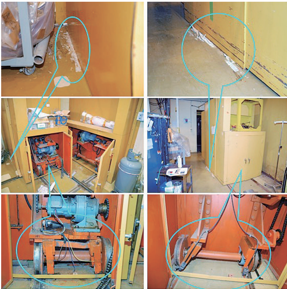
Fig. 7. Damaged shielding door. Drive component was completely destroyed, and main body of the door fell onto the floor. The doors blocked the entrances to the target rooms and made it impossible to bring in heavy machinery needed for the restoration work.
